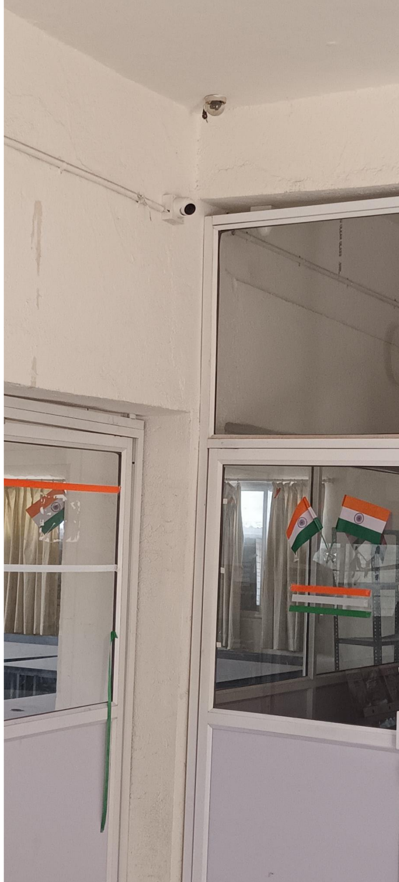
CCTV CAMERA'S IN COLLEGE LIBRARY
